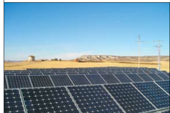
▲ Installation with Grupo Enepal in Spain
