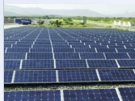
Xantrex installation, Ikea, Spain (Abasol).
