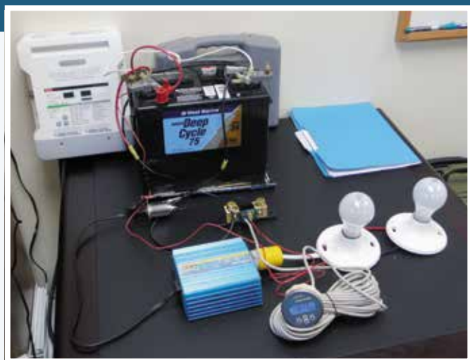
A Victron monitor is put through its paces. Two 70-watt light bulbs, powered through an inverter, created the load.
