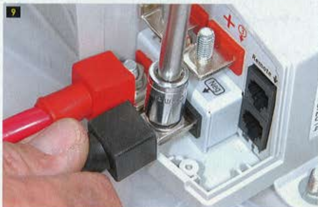
[8] Professional-grade cable crimpers are used to install terminals for connecting to the batteries. [9] Battery cable terminals are attached to studs that are found under the cover plate on the other side of the charger.
