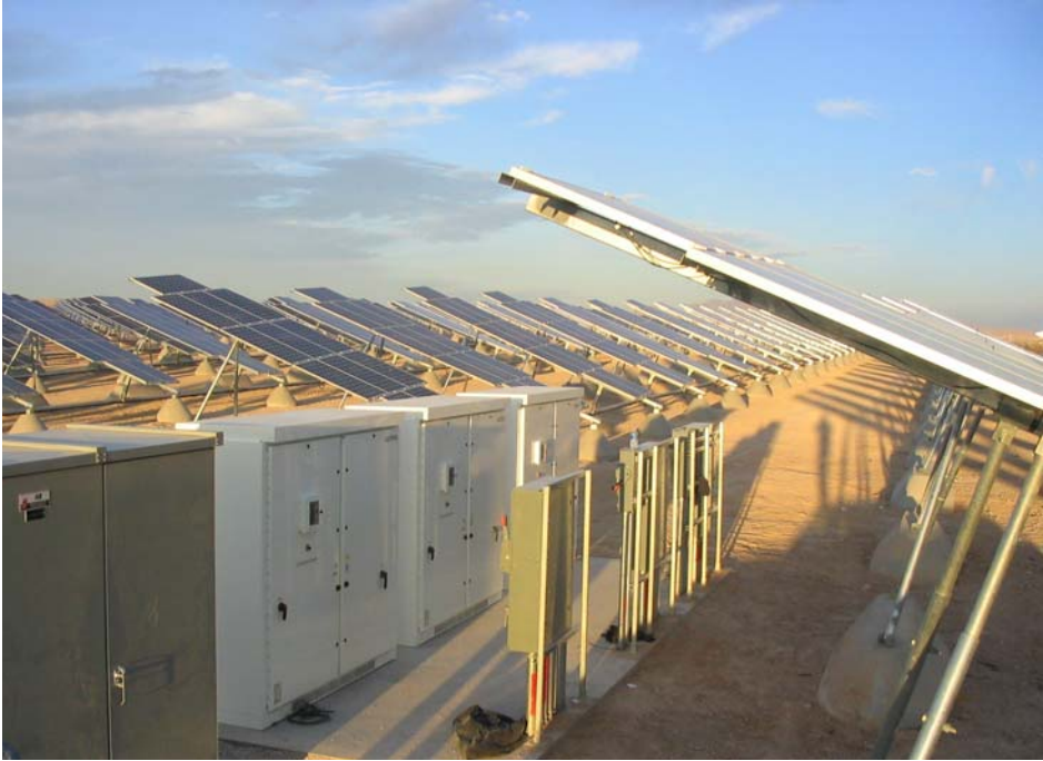
Xantrex inverters at the solar PV installation at Nellis Air Force Base, Nevada
